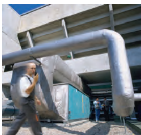
Air handling unit
