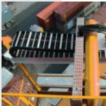
Wampfler Cobra energy guiding chain on a port crane.
